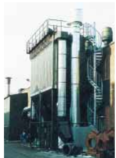
Filtering plant for flame cutting
